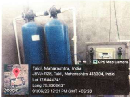
RO Water Treatment Plant
