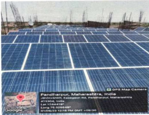
75 kW Solar Rooftop Plant
