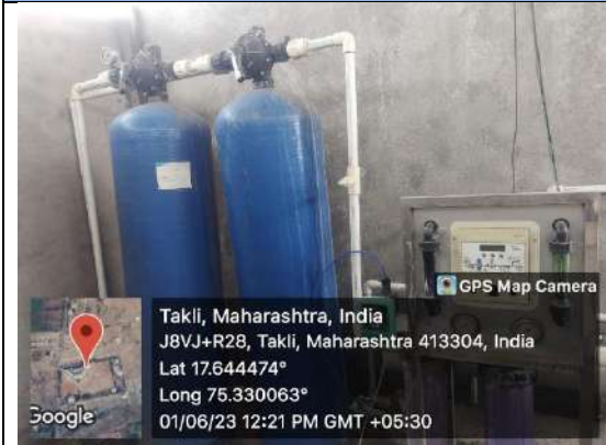
RO Water Treatment Plant
