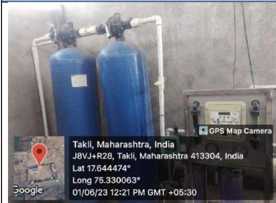
RO Water Treatment Plant
