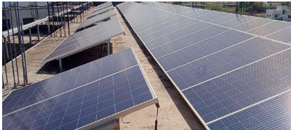
Roof Top Solar Power Plant which is working with capacity of 75 kW
